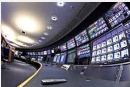
View of the control room of SES Platform Services.
